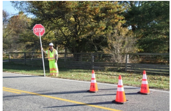
An example of Class 3 reflective wear requirement for flaggers and placement of three cones 15 feet or more in front of the flagger position.
